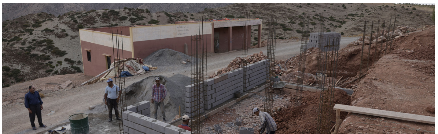
Reconstruction work in Al Haouz continues at a steady pace. Thanks to the consistency of contributions to the Fund created by the Government and to good governance, emergency support for earthquake-stricken populations has exceeded expected results (Photo by Bziouat)
